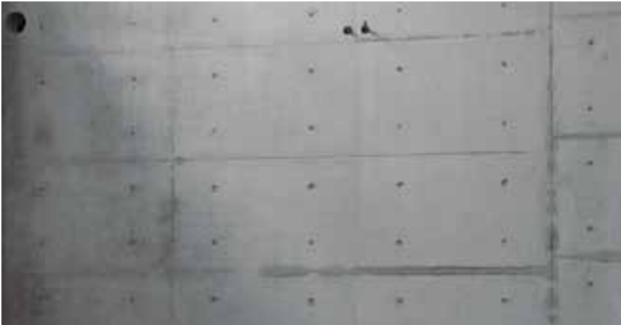
Dark discoloration on the plywood sheet/panel joint and the tie points. These areas are not sealed.
