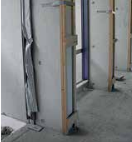
Edge protection directly on fresh concrete. Results in dark streaks on the corner of the concrete surface.
