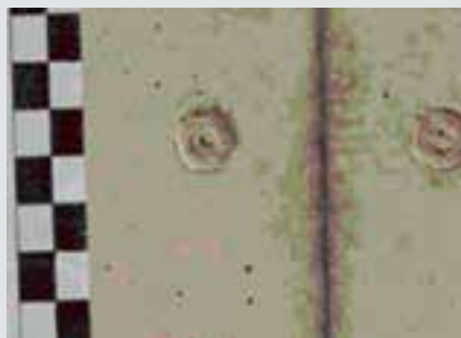
Impression of the staples on the concrete surface. Formlining: smooth, film-coated plywood sheet.
