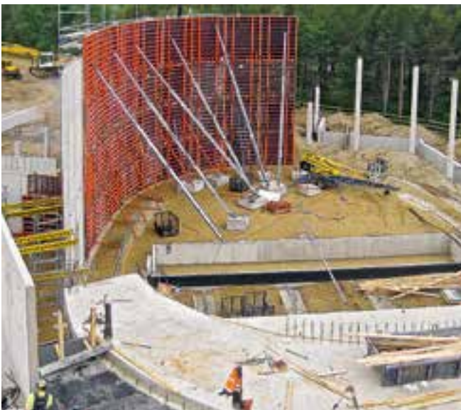
Curved walls of a container formed using TRIO elements with trapezoidal strips inserted in the joints.
