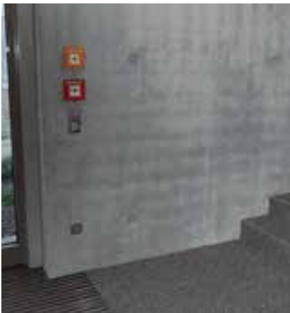
Wall reinforcement showing through. Prolonged contact of the internal vibrator with the reinforcement.
