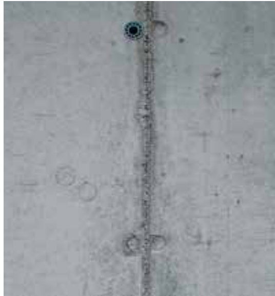
Element joint without any additional sealing, tie holes closed with plugs
