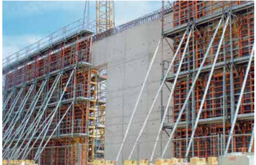
Concrete wall formed with PERI TRIO taken from the rental park; Formlining Class FC 1
