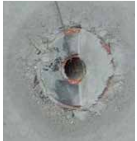
Bleeding in the area of the cone. Anchor not properly tensioned or non-elastic sealing rubber.
