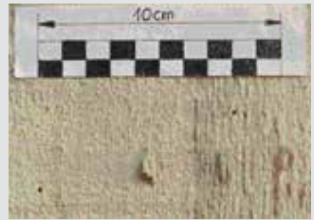
Fixing board formwork with staples. Impression of the staples on the concrete surface.
