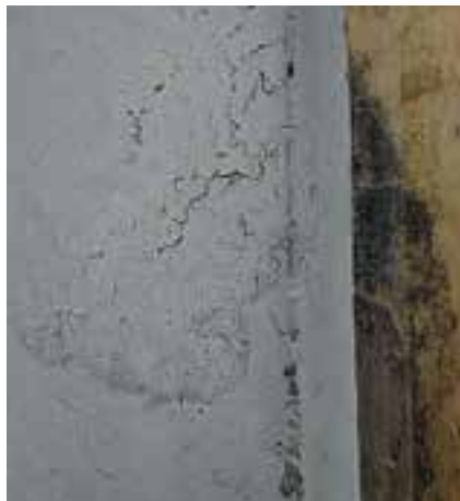
Aggregate nest. Incorrect vibrator handling.
