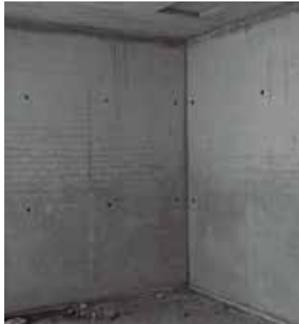
Lower half of the wall is darker than the upper half. Below: increased depositing of calcium on the concrete surface. This results in a thicker joint and thus in a darker appearance.
