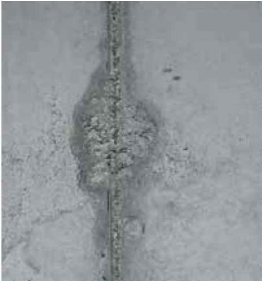
Panel joint without any additional sealing, leakage of fine particles possible!
