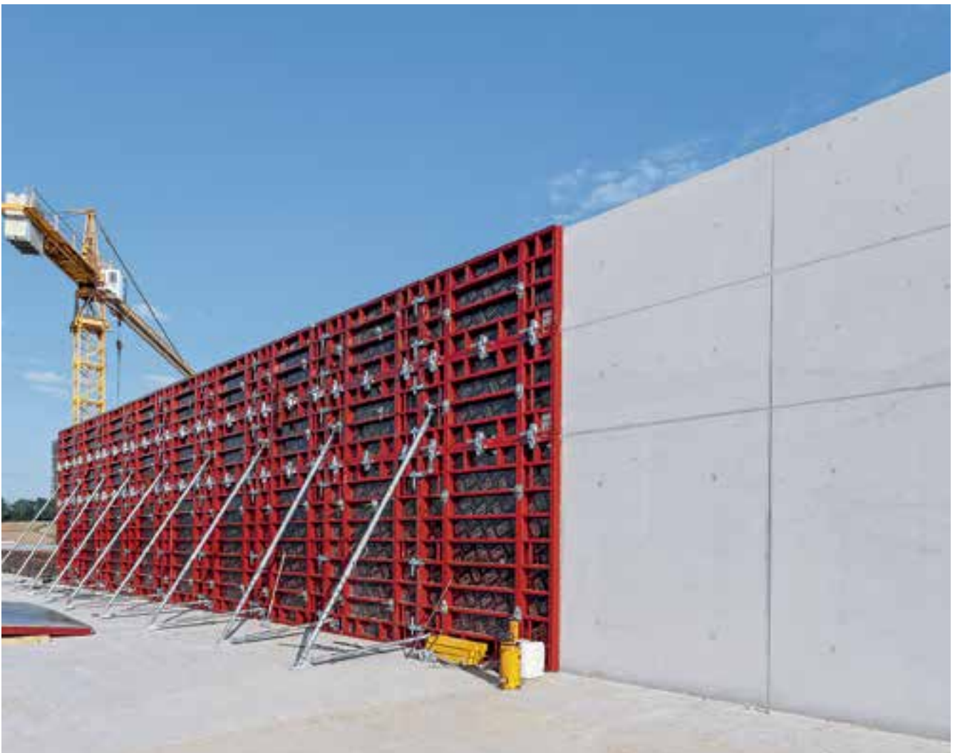
Concrete wall formed using PERI MAXIMO. Panel fitted with new formlining. Architectural Concrete Class 2
