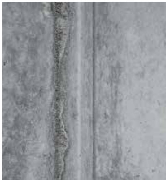
Details from left photo. Formlining/edge angle joint on the internal corner element
