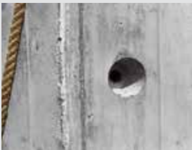
Element joint impression of girder formwork
