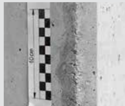
Here, the chamfer strip has been nailed to the stopend formwork. Due to the elongation of the anchors, a gap is created between the formlining and stopend formwork. The chamfer strip no longer seals. Ultrafine/ fine particles escape. (concrete bleeding)
