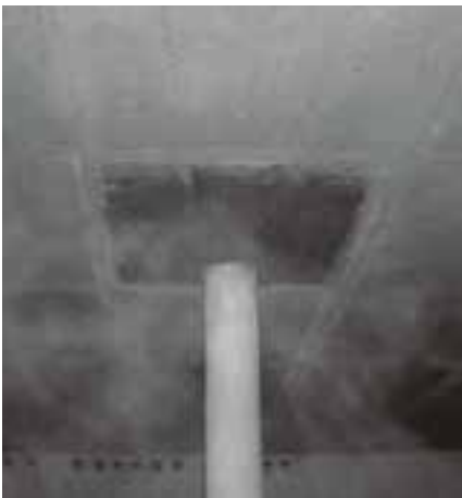
Dark discolouration on a slab soffit. Separating layer for slab prop made of wood materials or wood. Exchange of moisture between concrete and separating layer. Better to wrap the separating layer with geo-textile or foil.
