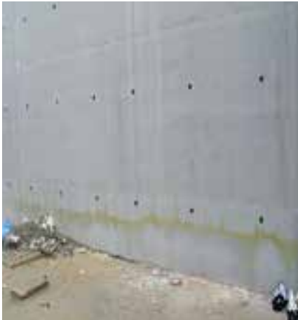
Brown/yellow discolouration. Condensation water with release agent residues.
