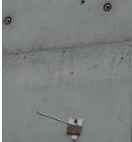
Air pores in the upper wall area. Post-compaction not carried out.
