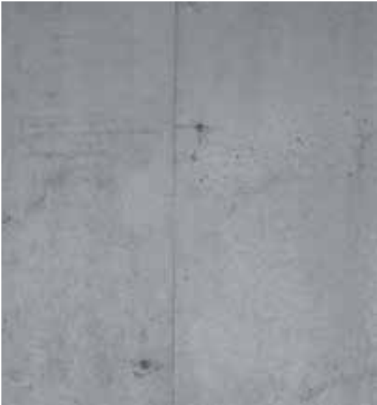
Large panel, formlining sheet central joint with rivet impressions, nailed to Structure
