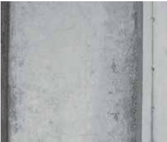
Stopend formwork used in the panel formwork, bevelled edges using timber chamfer strip
