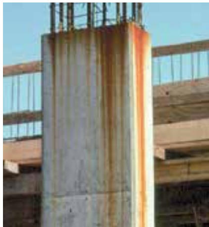
Rust streaks. No protection of the connecting reinforcement.
