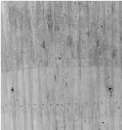
Light/dark discolouration of the concrete. The light area was covered during interim storage, the dark area exposed to the sun.
