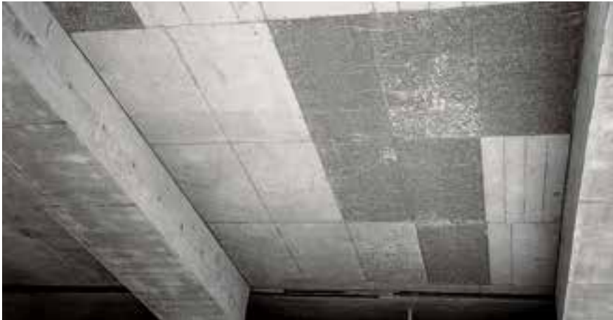
Slab soffit formed using different formwork panels (different surface structure, different absorption properties)
