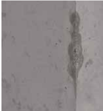
Sharp-edged corner with bleeding as a result of slight leakage on the formlining joint
