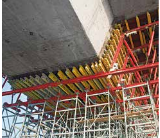
PERI framed formwork units were fixed to the bridge superstructure. In so doing, the shoring construction could then be sectionally dismantled for the next cycle.
