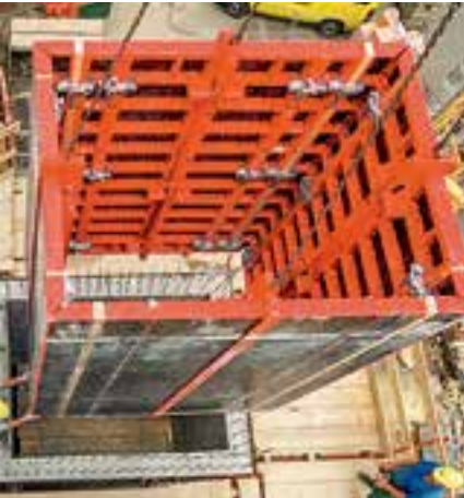
Rectangular shafts require adjustable crane slings due to the different lengths of the attachment points. This results in approximately the same tensile force on all four slings.
