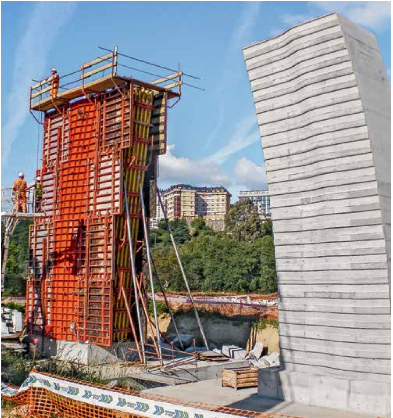
TRIO Structure being used to form a bridge pier: being covered with additional strips of wood results in an interesting surface structure.
