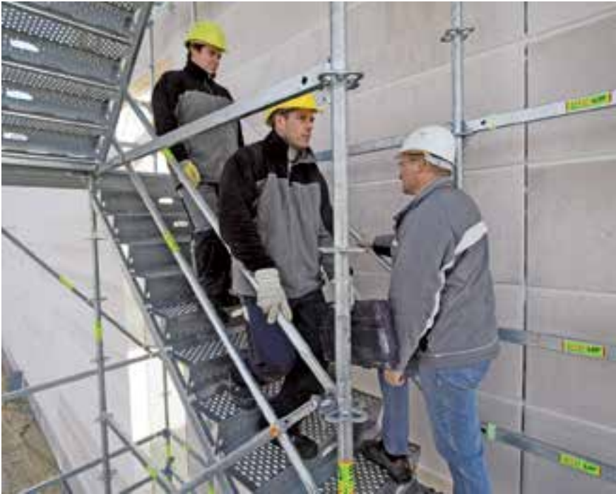
The stair width of 100 cm is easily accessible with sufficient space for site personnel to pass each other as well as for rescuing injured persons.
