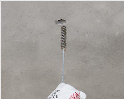
Step 1 Drill hole with d = 22 \text{ mm} and t = 160 \text{ mm} (at right angles to the concrete surface); clean the drilled hole with brush and blow-out pump
