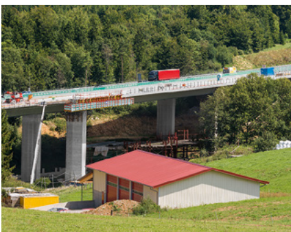
During the bridge construction work, traffic on the A 81 motorway was able to use the already completed superstructure between the Geisingen and Engen junctions.
